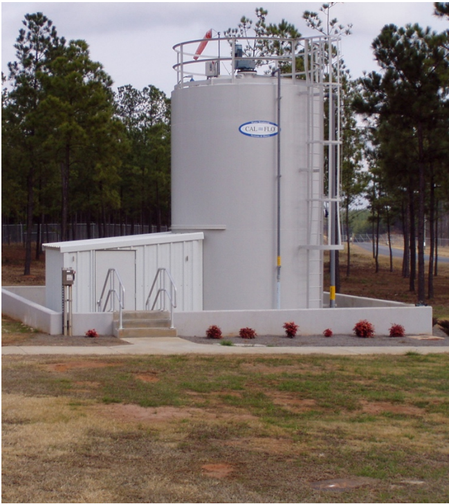
Figure 1. CalFlo Liquid Lime System by Burnett Lime Company, Inc.
